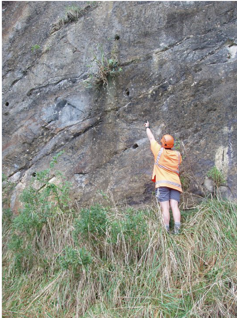
Figure 7: Karen Rohloff points to the water stain below one of the exploratory holes drilled into the western end of the quarry face around 2000. The water stain is an indicator that there is space – a cave- behind this end of the quarry wall. Photo: Mary Traves, 2013
