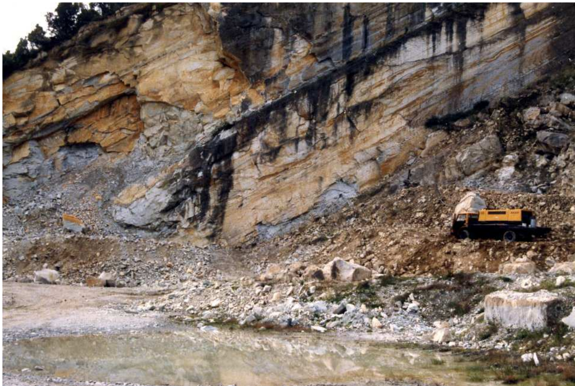
Figure 6: Preparatory drilling being carried out in the mid-quarry area in 1986. The drilling rig is near the face on the upper bench with a compressed air line running up to it from the compressor truck. Note the unstable area with overhang and arch, the result of blasting in November 1984. Photo: WCRC Collection
