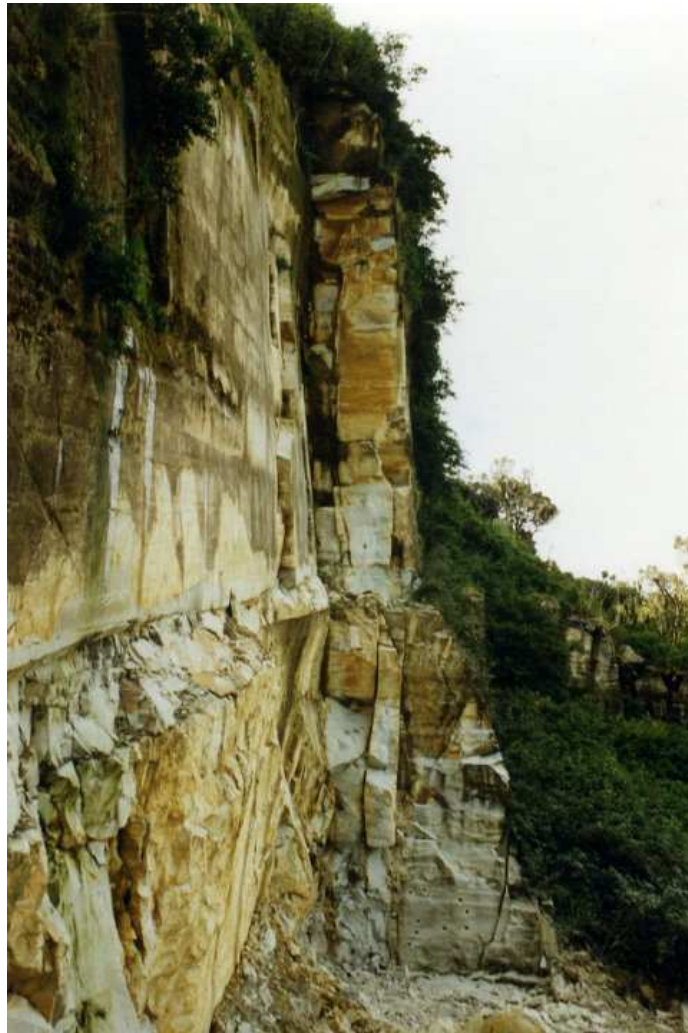
Figure 5: View along the quarry face looking east taken in the 1990's at the time of drilling for a small blast. Note the mudstone band at the point of the slight bulge in the quarry face. Photo: Graham Warriner
