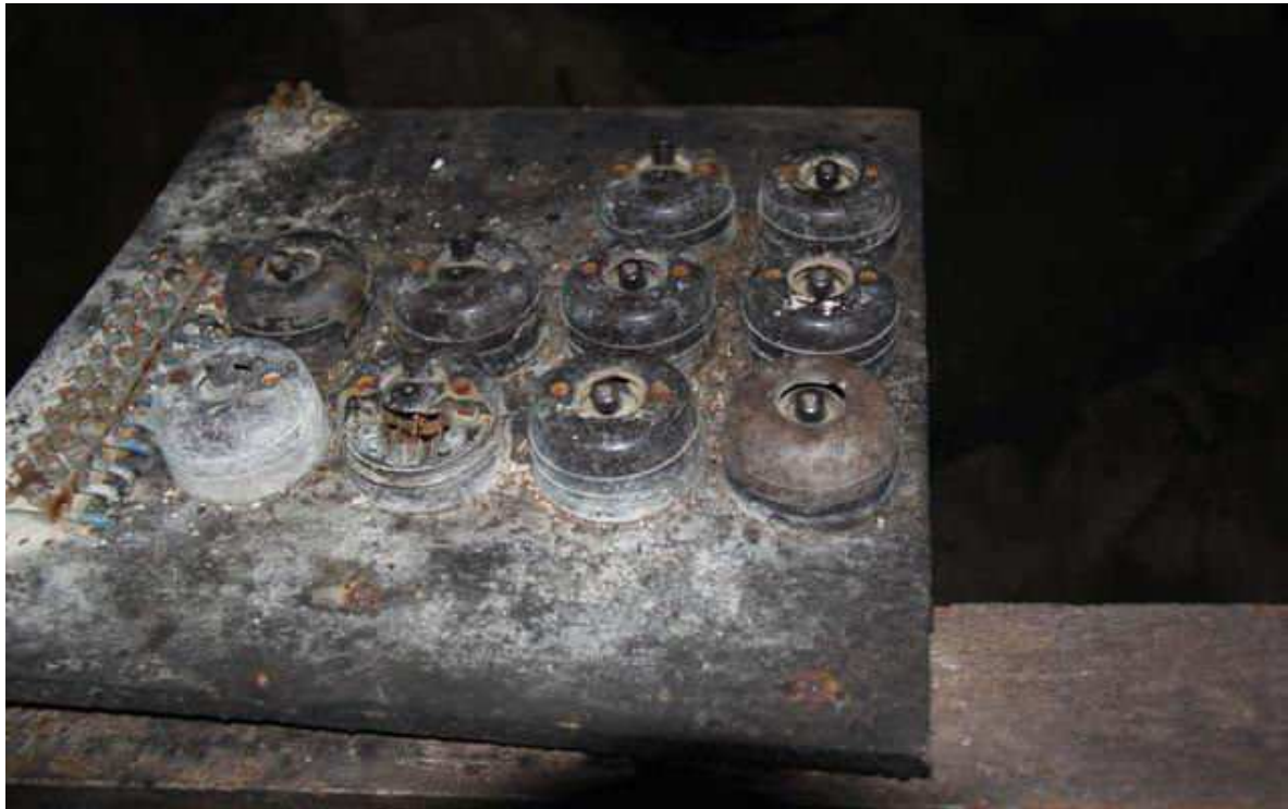
Old switch boards installed in 1970s and used into the 21 st century
