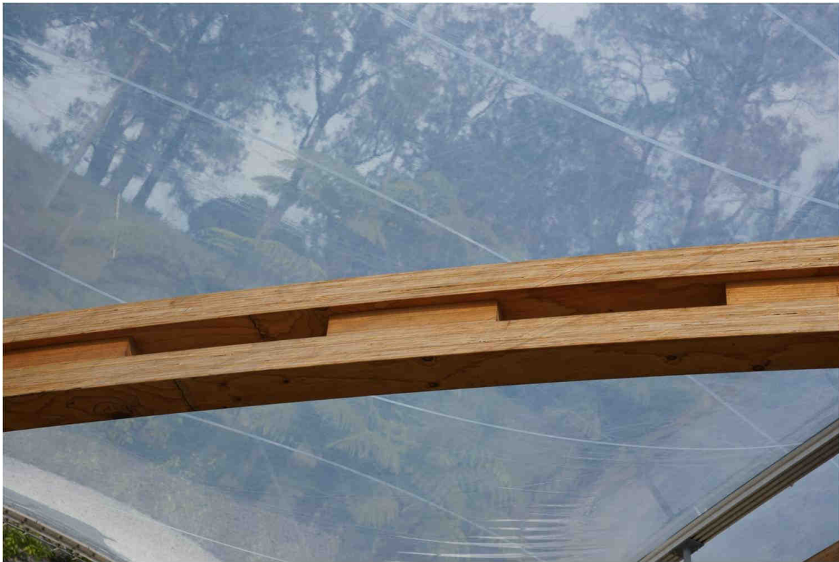
Efte (teflon) inflated pillows provide the roof canopy
