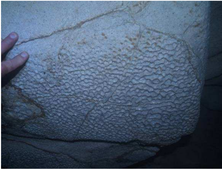
Figure 3b) Example of condensation corrosion in the Organ Loft caused by historical high CO 2 levels (before real-time monitoring and ventilation management)
