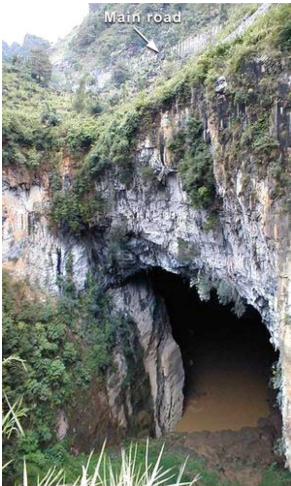
Figure 23: The 200m deep Yanliu Dong collapse doline, south of Lingyun County town; arrow points to position of main road built on top of a 15m high vertical retainer wall where road traverses steep cone karst hillside above the collapse feature.
