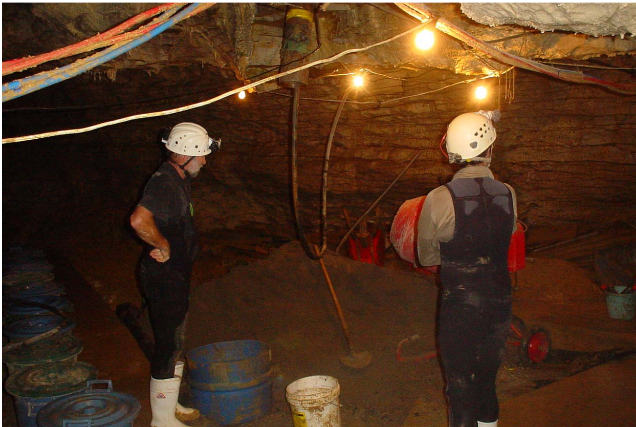
Van Watson and Pete Chandler at the main works site in Ruakuri Cave. Note the bottom of the drilled pipe for bringing concrete into the cave (centre top of photo).
