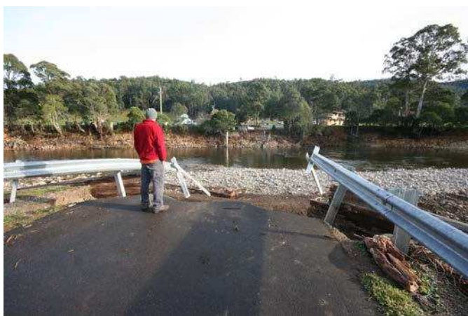
Liena Bridge on the Mersey River – destroyed during the flood
