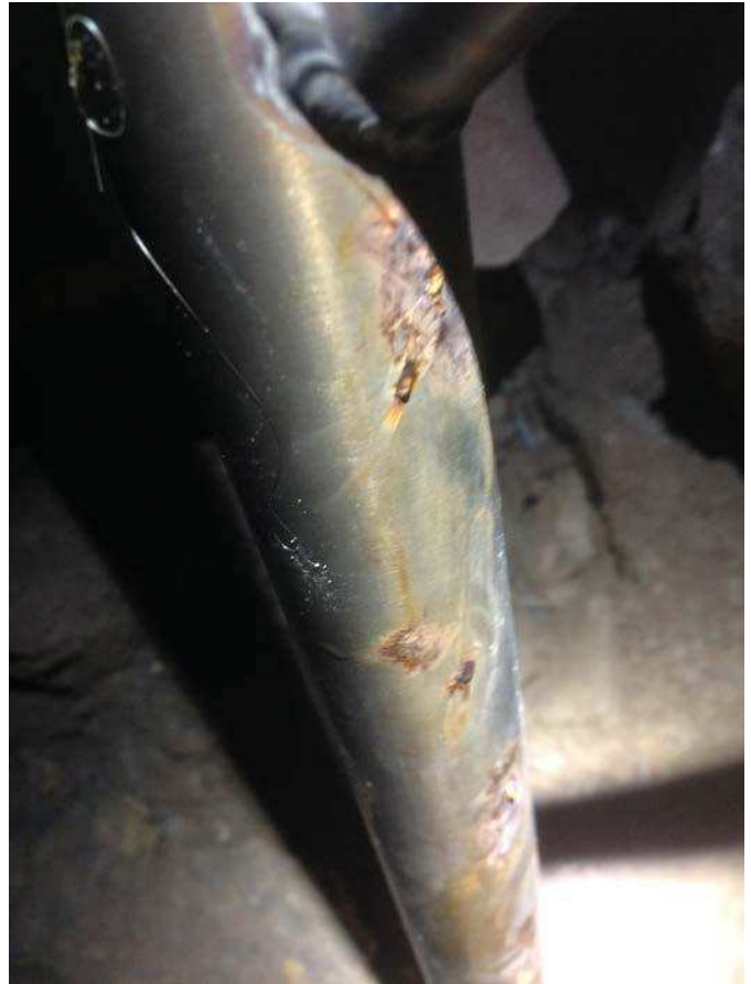
Severe rusting on the brown stainless steel in River Cave
